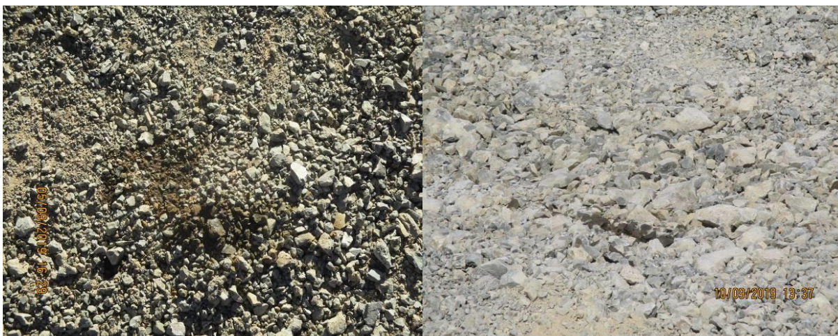
Photo: Oil spill (laydown area).
