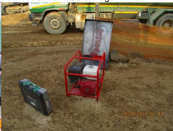
Photo: generator on the ground with drip tray
