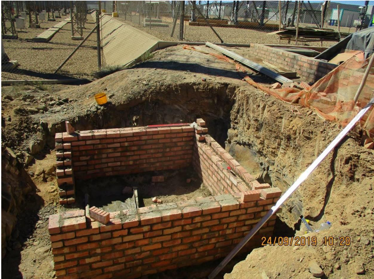
Photo: Construction of bund for oil water separator at the servicing area.
