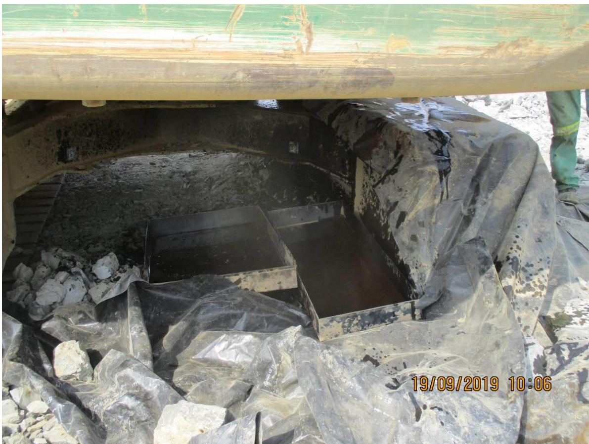
Photo: Moderate oil spill due to hydraulic pipe burst from excavator (BWX 13).
