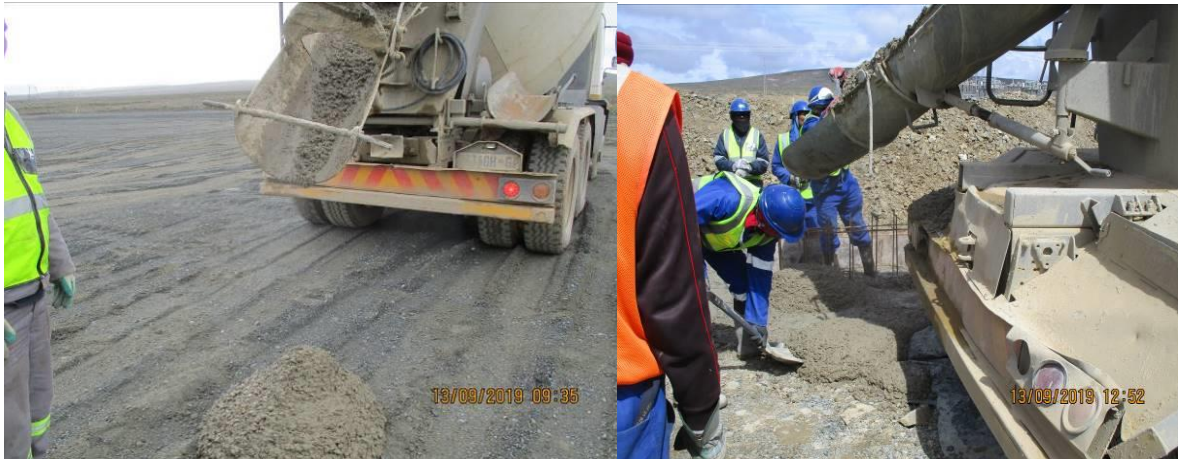
Photo: Concrete spill at 132kV terrace (section A) during concrete works at the retaining wall
